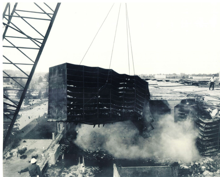
Steel shelving being removed through the collapsed ceiling.
