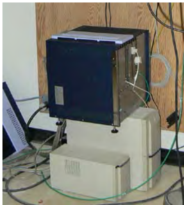
Figure 6. PBX balanced on top of UPS
