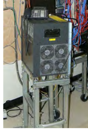
Figure 5. Switch on temporary rack
