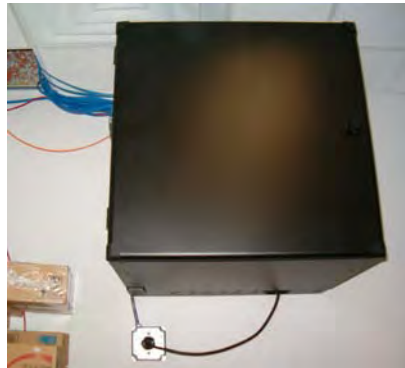
Figure 3. Rack was unlocked and key was located on top of the rack
