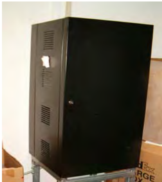
Figure 2. Rack was unlocked
