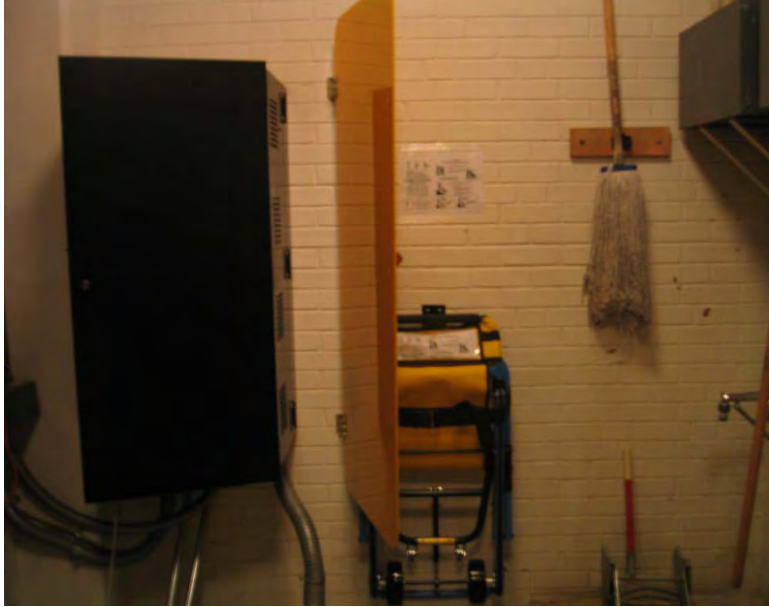
Figure 1. Network equipment stored in Janitorial Closet
