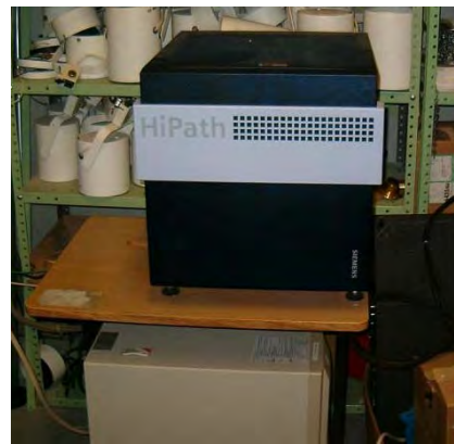
Figure 7. PBX not in a rack
