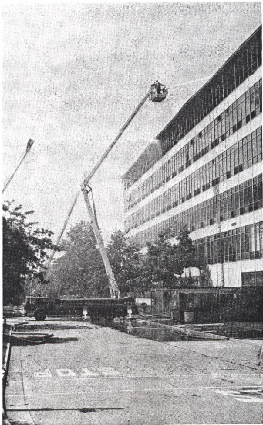
Fire department snorkels fighting the fire. Note the outward deflection of the sixth floor curtain wall.
